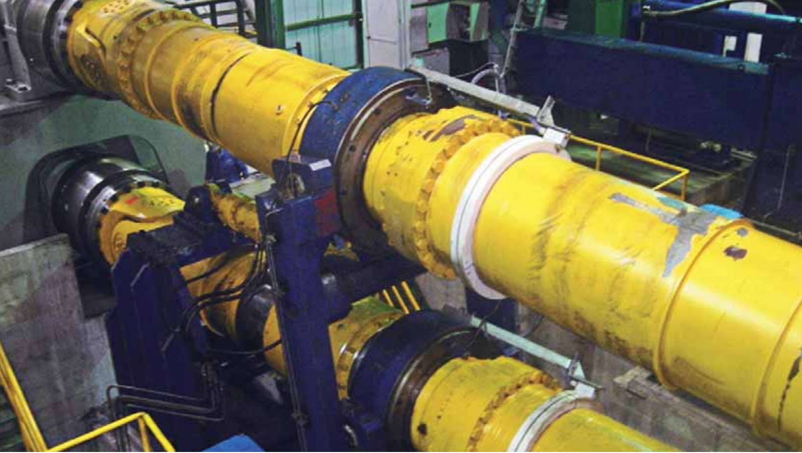
Torque measuring in a steel mill driveline.
