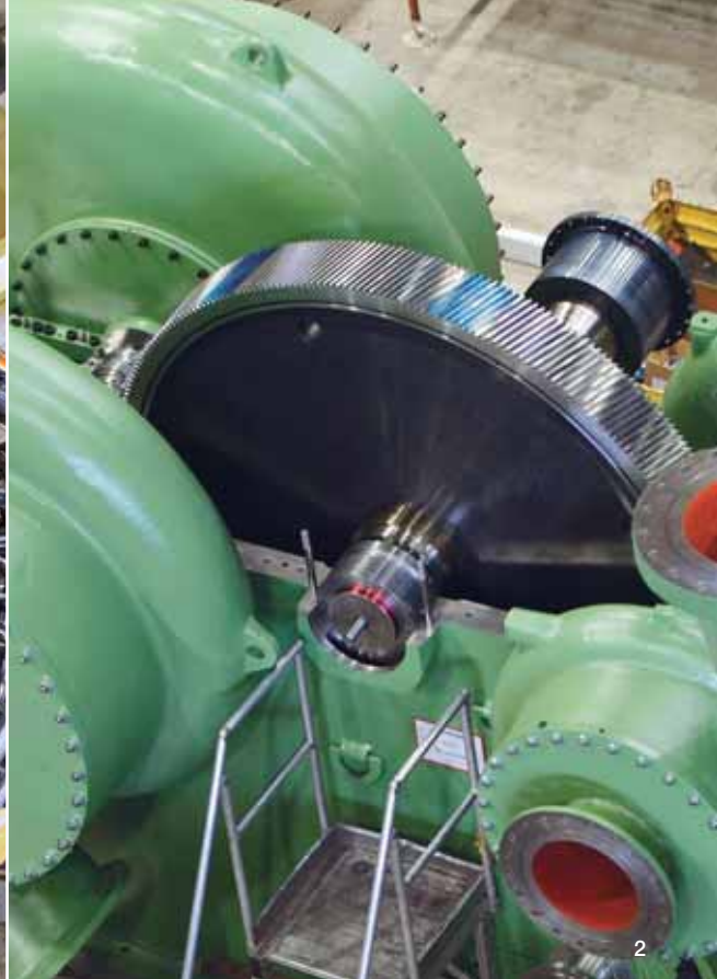
1 GE LM 6000 Gas Turbine 2 Siemens Compressor
