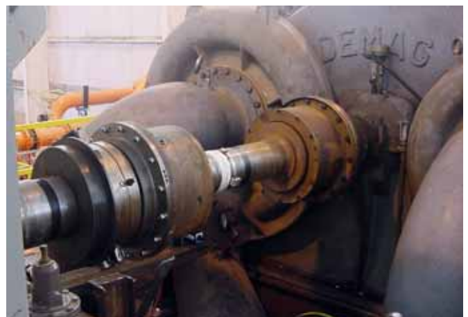
SmartSet retrofit in a 8000 HP Compressor
